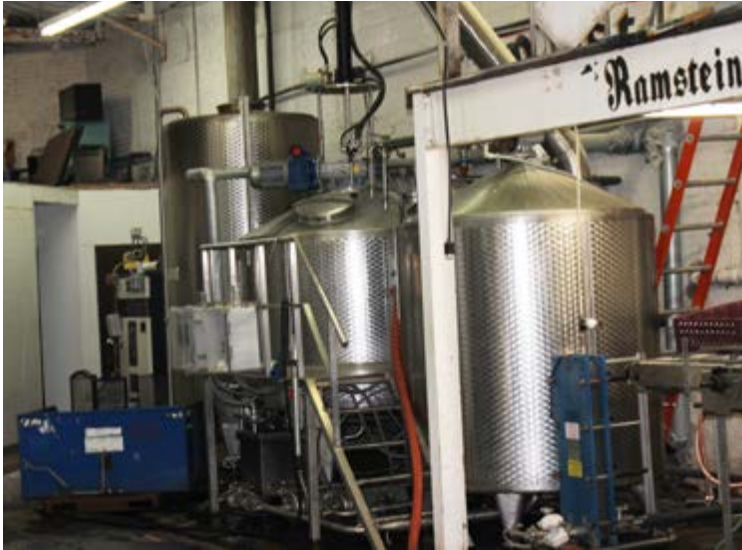
Hot Liquor Tank and 15 BBL Brewhouse
