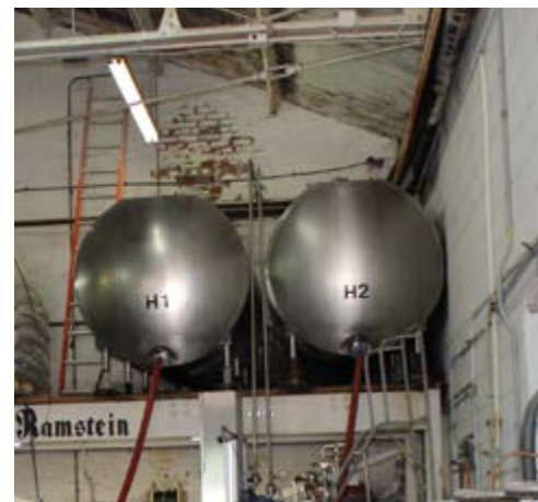
Horizontal Brite Tanks
